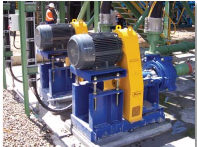
Jebsen & Jessen Technology's WMA pumps operating in a gold mine in Indonesia.
